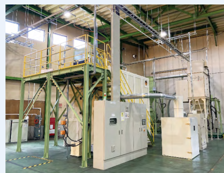
Crushing and separation facilities
