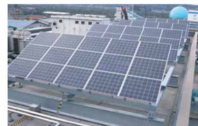
Solar power system at the research and development center
